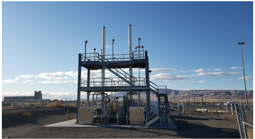
EM’s Office of River Protection and tank operations contractor Washington River Protection Solutions continue to enhance safety in the Hanford Site’s Tank Farms with the completion of a new exhauster ventilation system in the SY Tank Farm. All six of Hanford’s double-shell-tank farms are now ventilated by upgraded exhauster systems.
