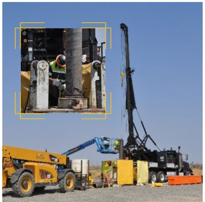
EM contractor Central Plateau Cleanup Company is installing more than a dozen additional extraction wells this year to support expansion of the Hanford Site’s largest groundwater treatment facility.
