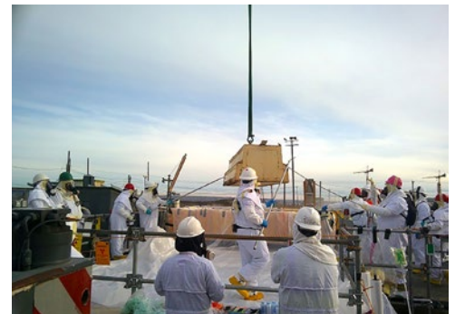
Crews safely remove legacy equipment from the Hanford Site's A Farm to prepare for future waste retrievals.
