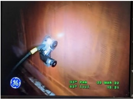
A mini crawler, developed by Florida International University students and faculty, moves along the outside of the inner tank shell on a double-shell waste-storage tank at the Hanford Site.
