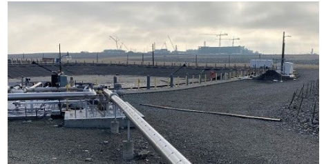
During Hanford’s Direct-Feed Low-Activity Waste Program treatment operations, the Waste Treatment and Immobilization Plant, background, will feed liquid waste to the Liquid Effluent Retention Facility, foreground, through this primary transfer line.
