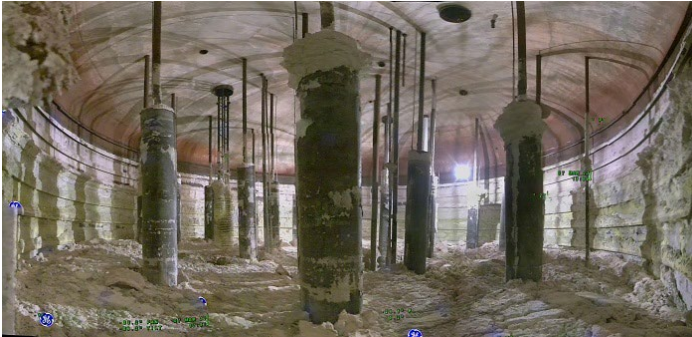
Waste retrieval from Tank AX-101, the last of four tanks to be retrieved in the Hanford Site's AX Farm, is set to begin this fall. This in-tank photo shows the salt-based waste and the tank's 22 air-lift circulators.
