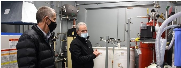
Brian Vance, manager of the Office of River Protection and Richland Operations Office, left, is given a tour of the Tank-Side Cesium Removal (TSCR) system ancillary enclosure by John Eschenberg, president and CEO of Washington River Protection Solutions.
